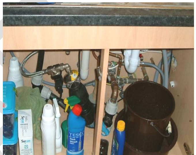
Example of poor installation, with no marking to clearly identify rainwater from mains water.
