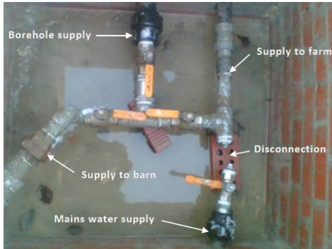
A cross-connected borehole supply pumped un-wholesome water into the public mains supply (now disconnected) because of the difference in supply pressures.
